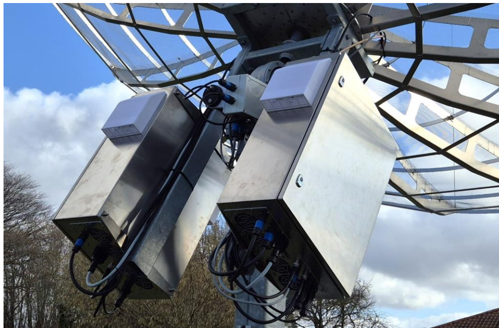
PA systems installed at dish
