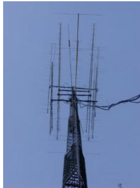
K1JT's antenna array includes yagis for 70 and 23 cm
