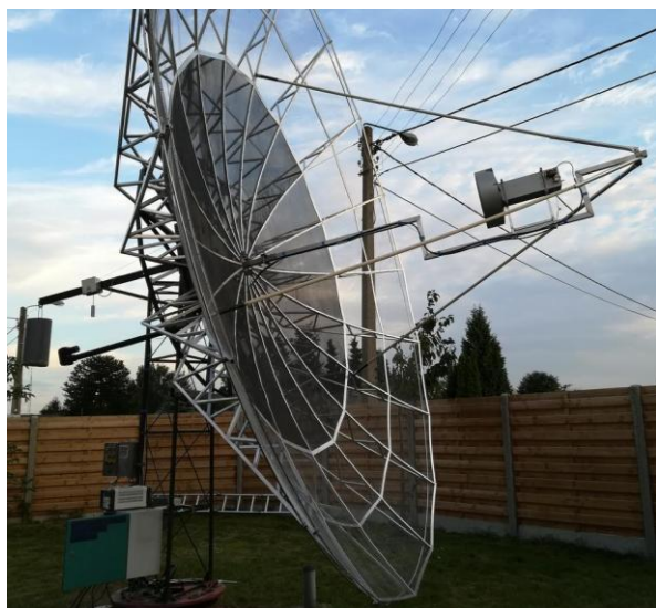
ON5GS's new 6 m dish - See QRZ.com for a detailed picture story of Dirk's dish construction
