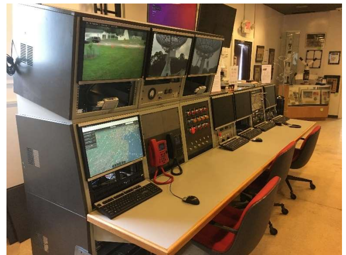
Figure 18- ISEC Control Center
