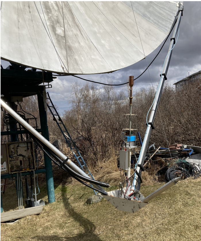
KL6M 10 GHz Rig Installed at Feedhorn
